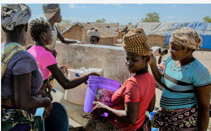
IOM constructs water points to provide access to water displaced and host community members. © IOM 2022
